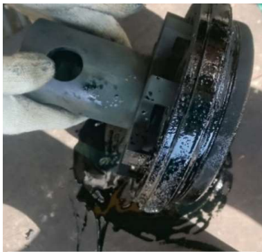
Sludge condition of current valve
