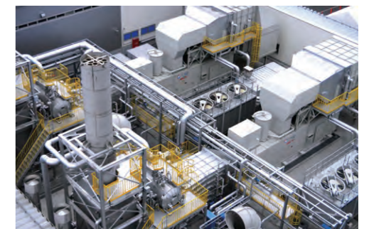
A gas turbine co-generation system
