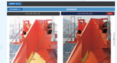
Image showing signs of age-related deterioration
