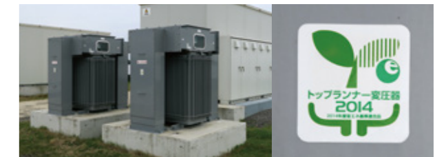
High-voltage transformers that conform to the Top Runner standards
