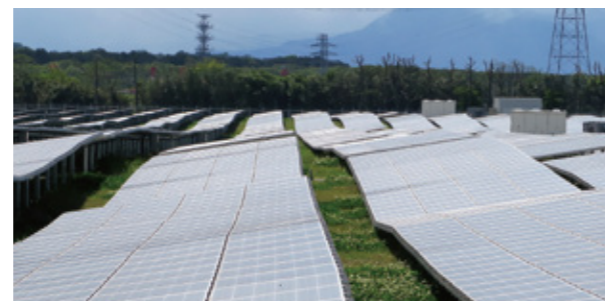
Solar panels set up on the existing rainfall slopes of the land
