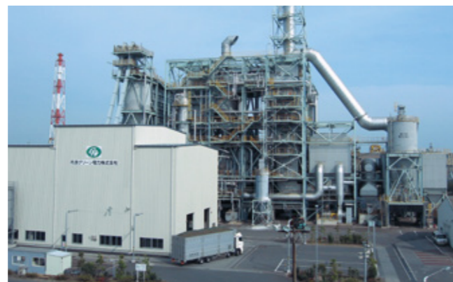
Power generation facility at Chiba Works of MES (Ichihara City, Chiba Prefecture)
