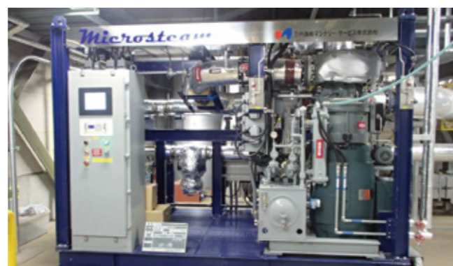
The small-scale steam power generation facility at Karatsu-shi Seisou Center
