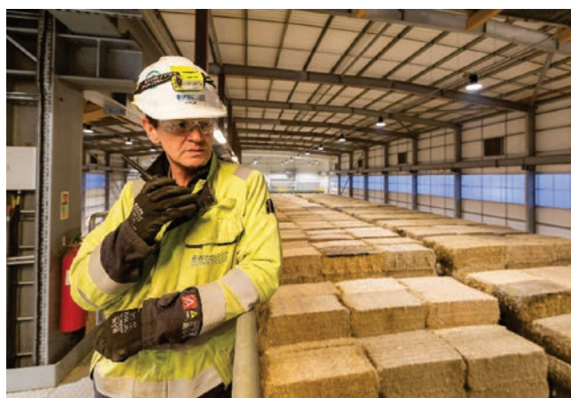
Photo 5 Operation and maintenance at Snetterton Renewable Energy Plant in the UK.
