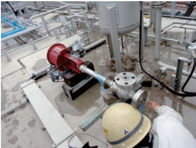
写真3 膨張弁解放検査の様子 Overhauling Inspection inside of Expansion Valve
