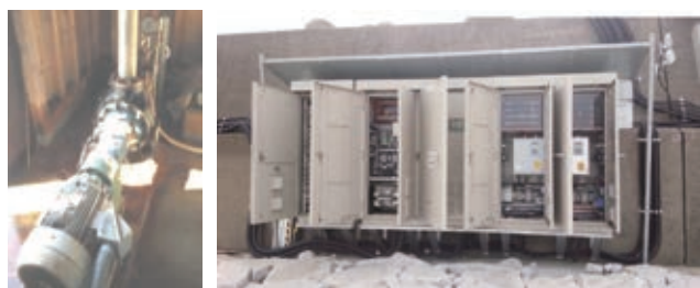
写真3 設備(左:汲み上げポンプ,右:新設の制御盤) Testing Facility on land(Left: Pump, Right: Controlling Panel)
