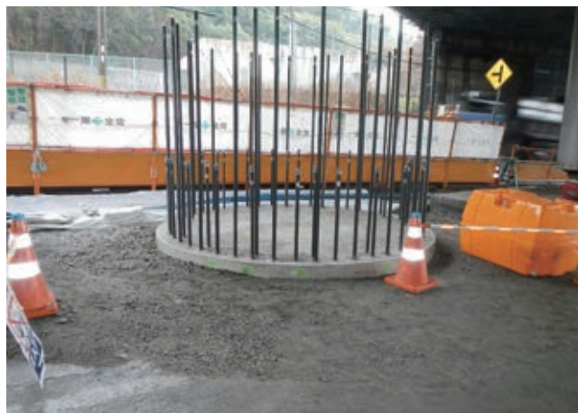
写真3 基礎工及びRC柱1次施工 Construction of Pier Foundation and Primary Construction of RC Pier
